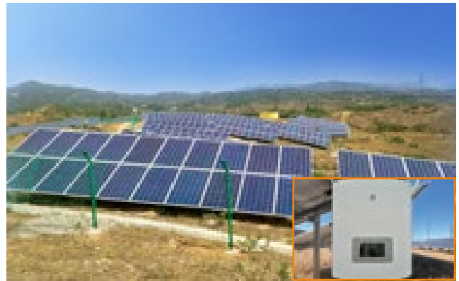
Hebei Qinghuangdao poverty alleviation PV Plant 9.7MW
