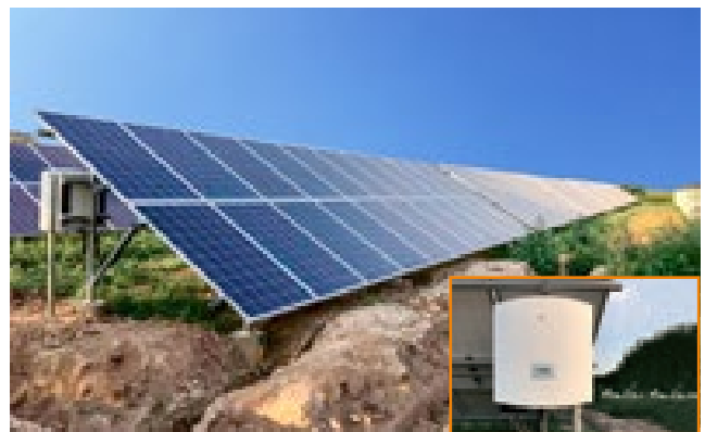
Hebei Qinghuangdao poverty alleviation PV Plant 5MW
