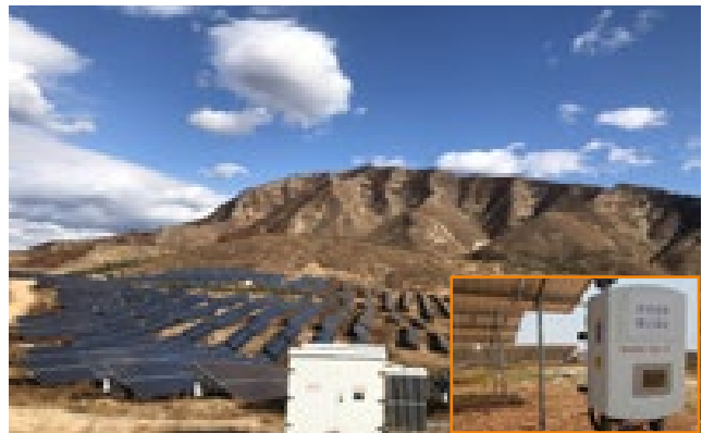
Liaoning Gaizhou Jiuzhai PV plant 20MW
