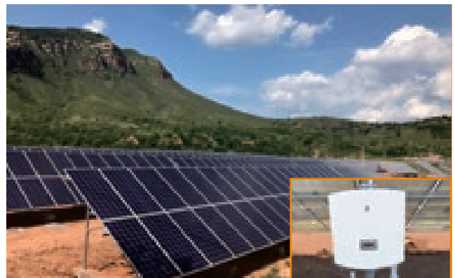
Shanxi Xiyang poverty alleviation PV Plant 7.2MW
