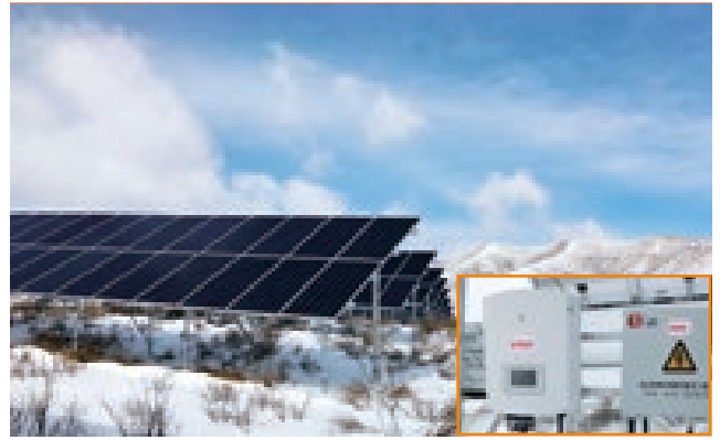
Shanxi Guangling PV plant 1.47MW
