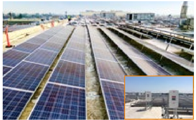
United States Postal Service (USPS) LA P&DC Facility, U.S.A 13MW
