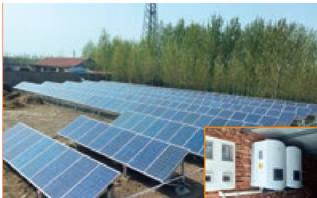
Shandong Leling poverty alleviation PV Plant 50kW
