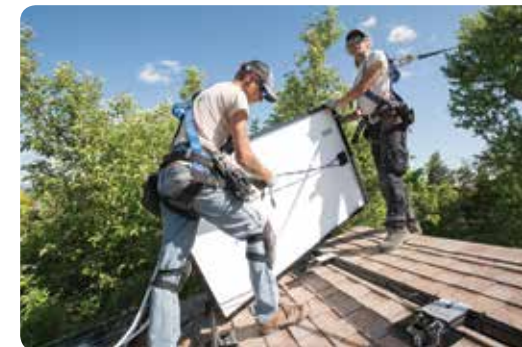
SolarEdge at home
